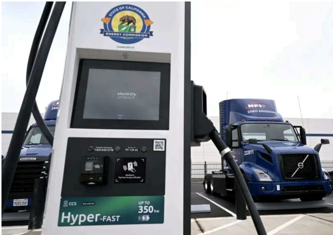
This February 2024 photo shows battery chargers and electric-powered semi-trucks at NFI's Ontario truck depot. A new study says more must be done to ensure the Inland Empire addresses infrastructure and other concerns as trucks transition from diesel engines. (File photo by Will Lester, Inland Valley Daily Bulletin/SCNG)
